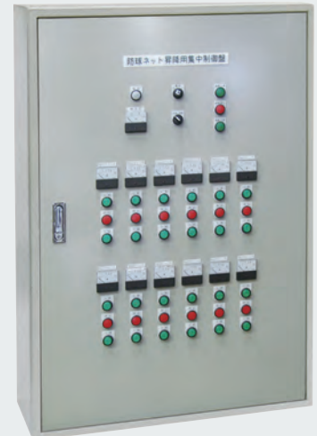
Centralized Control Panel
